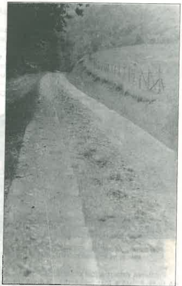
Foto 5. Vedere de ansamblu a tronsoanelor la doi ani după execuție. (General view of the roads two years after they had been put into execution).
